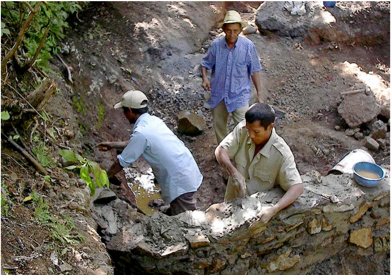
MCC Photo: Masons from Las Pozas and Las Lomitas, Honduras, work together to build a dam. In the foreground are Victorino, left, and Reyna, from Las Pozas. Behind them is Jose Leon, a member of the Las Lomitas Brethren in Christ Church. (Photo by Tony Sauder)
